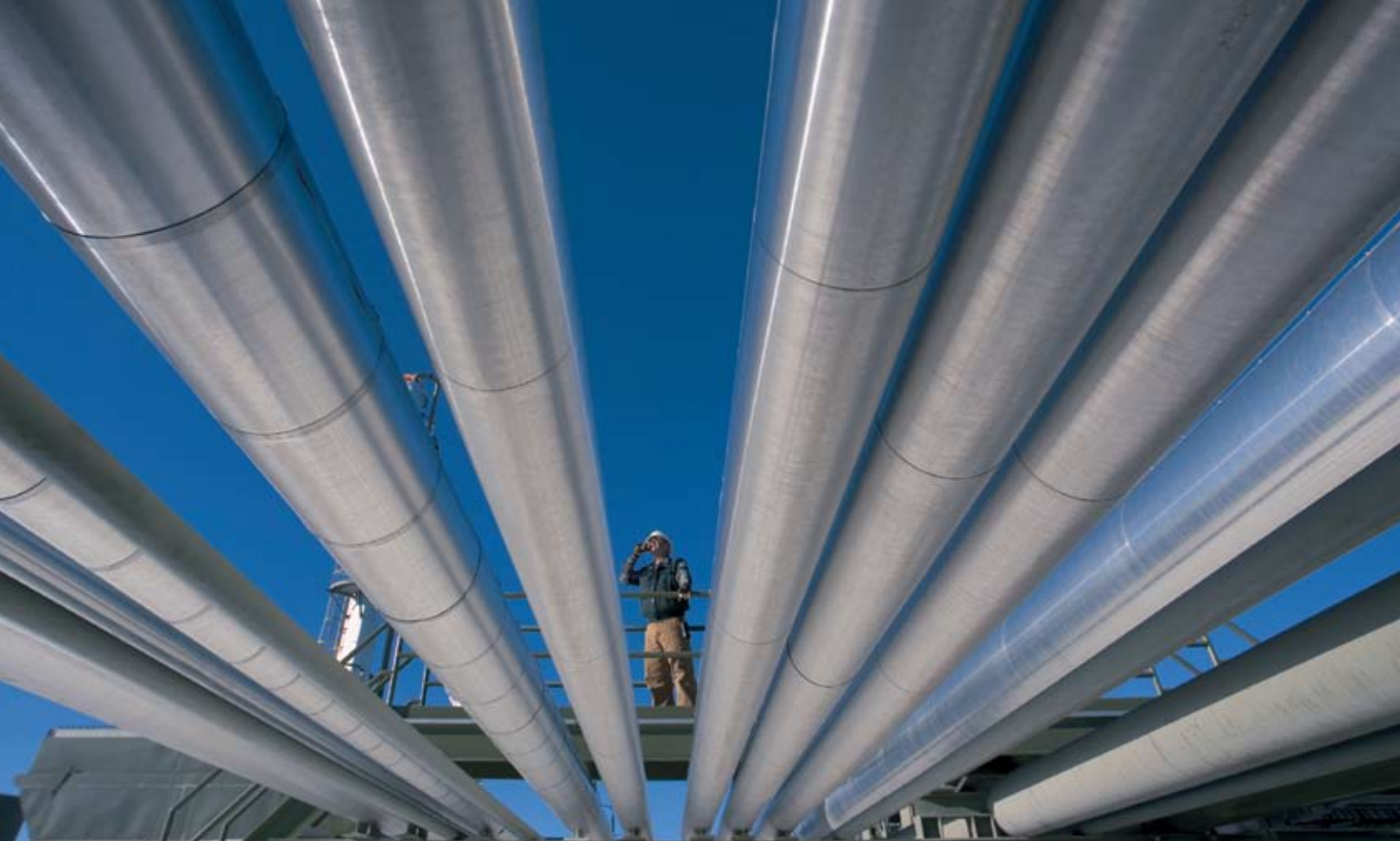
Bobby Schoggins, senior operator, makes sure the gas processing plant runs close to its capacity of 50 million cubic feet per day.
